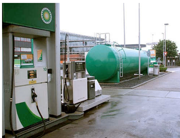
Figure 12: B30 fuel pump in Naaldwijk, The Netherlands
