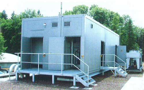
Plant for biogas conditioning built as a block (photo: Carbotech)
